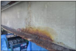
(a) corrosion member
