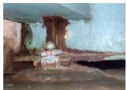
Fig. 1. Corroded girder end
